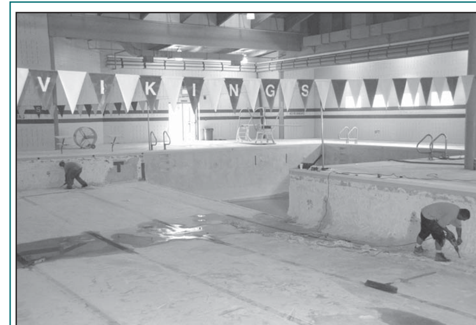
Workers use high-powered tools to resurface the Puyallup High School pool and pool deck over summer.
